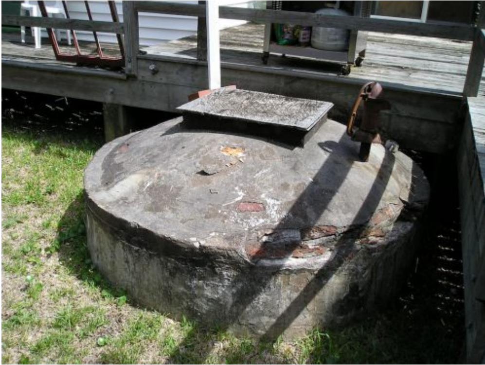
Cubicle Cistern "Down Point":
